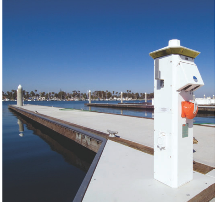
Lighthouse - SS Power Pedestal
