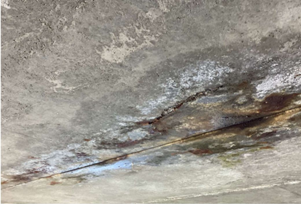
Delamination and Rust Staining in Underside of Slab
