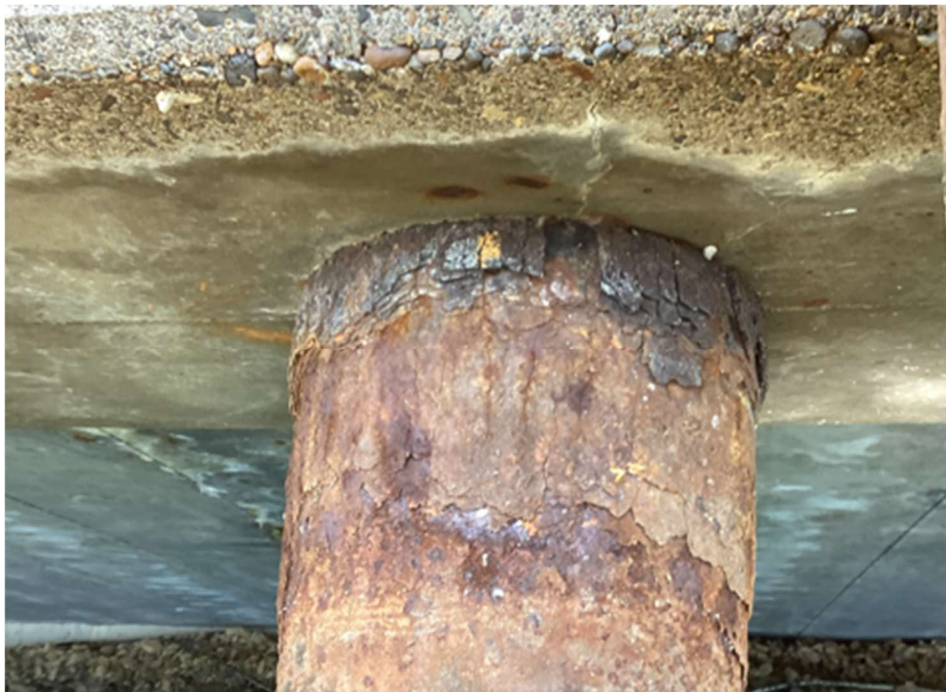
Pile Corrosion at the Cap Interface
