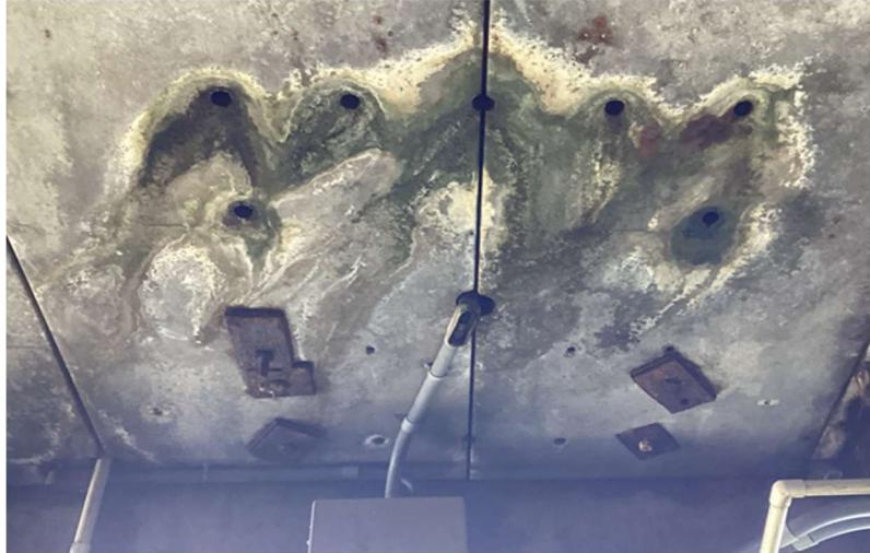
Holes in Slabs and Hoist Connections
