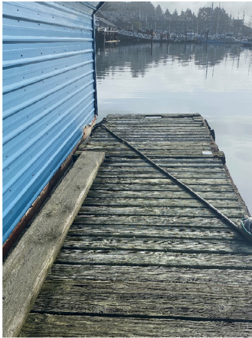
Photo 4: Supplemental rope restraining Dock B to nearby piling
