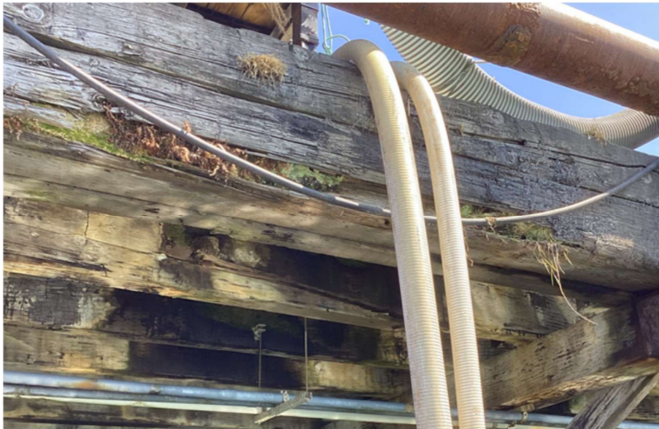
Broken Timber Girder
