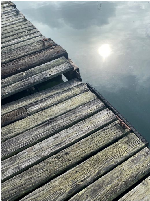
Photo 2: Missing hardware near space 15 on Dock B
