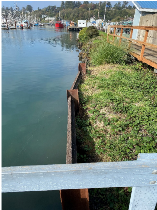
Photo 18: Leaning bulkhead wall
