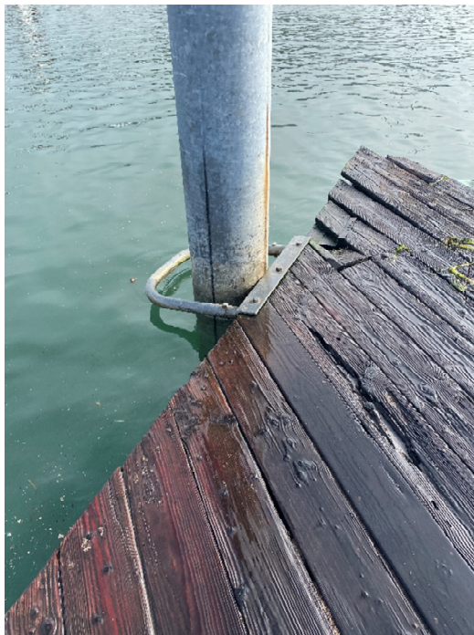
Photo 13: Typical pile hoop attachment
