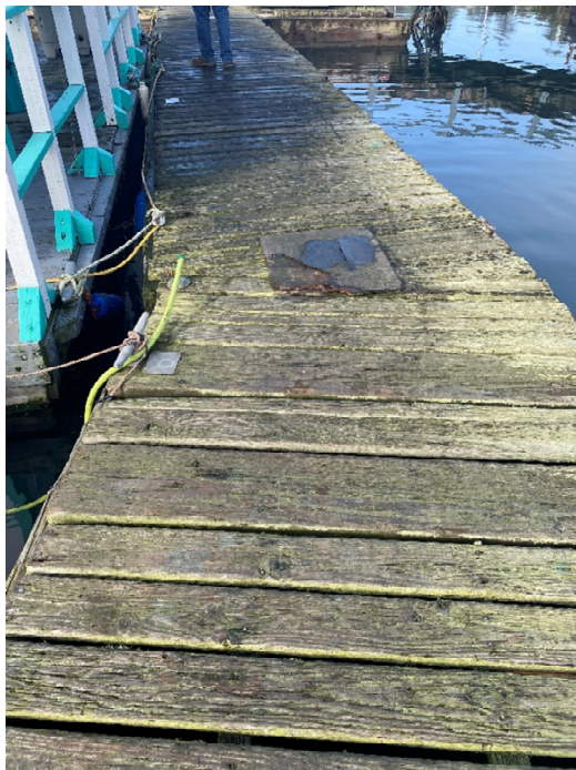
Photo 3: Hole with decayed patch in Dock B
