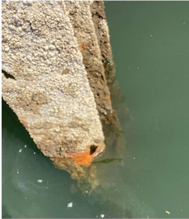
Fender Pile Corrosion at Waterline
