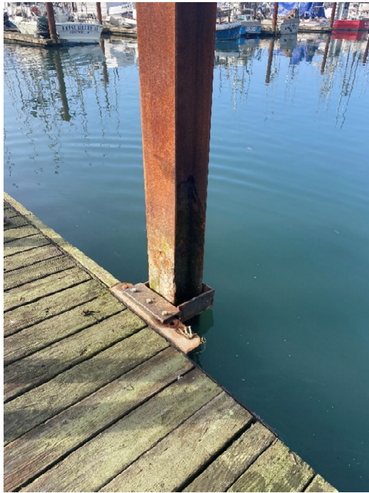
Photo 14: H Pile on Dock X near the gangway. Note heavy corrosion near the waterline.
