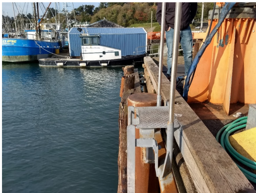
Photo 14 – Hoist Dock – Rotting Fender Piles
