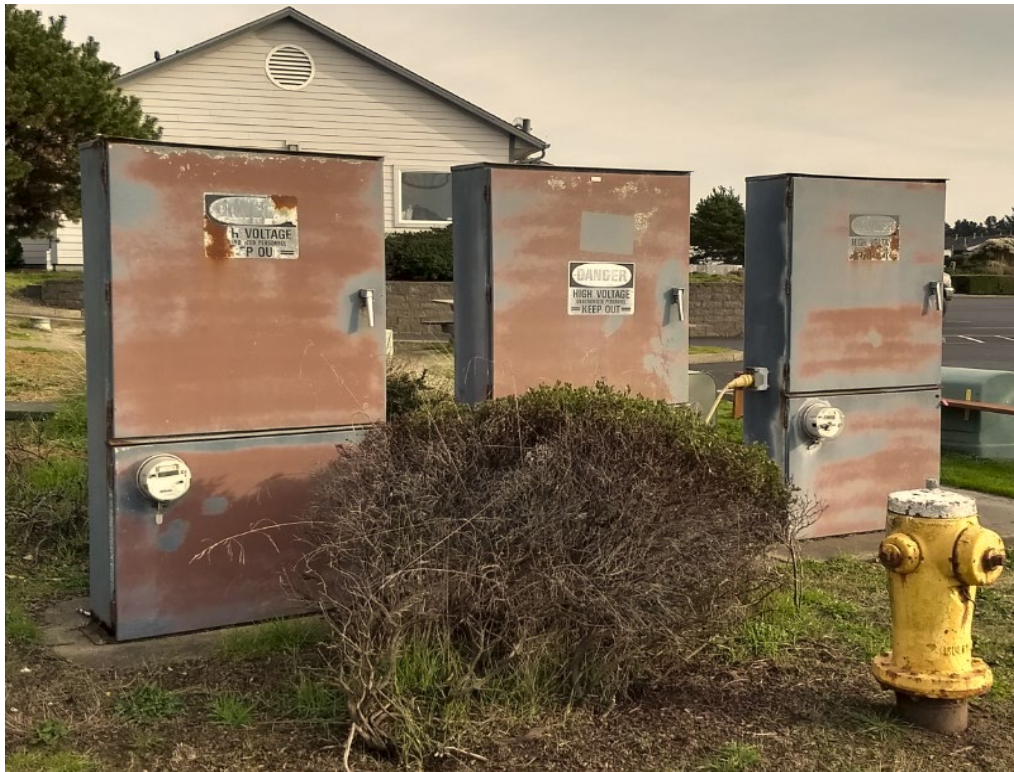
Photo 28 – South Beach Marina – Electrical Load Centers
