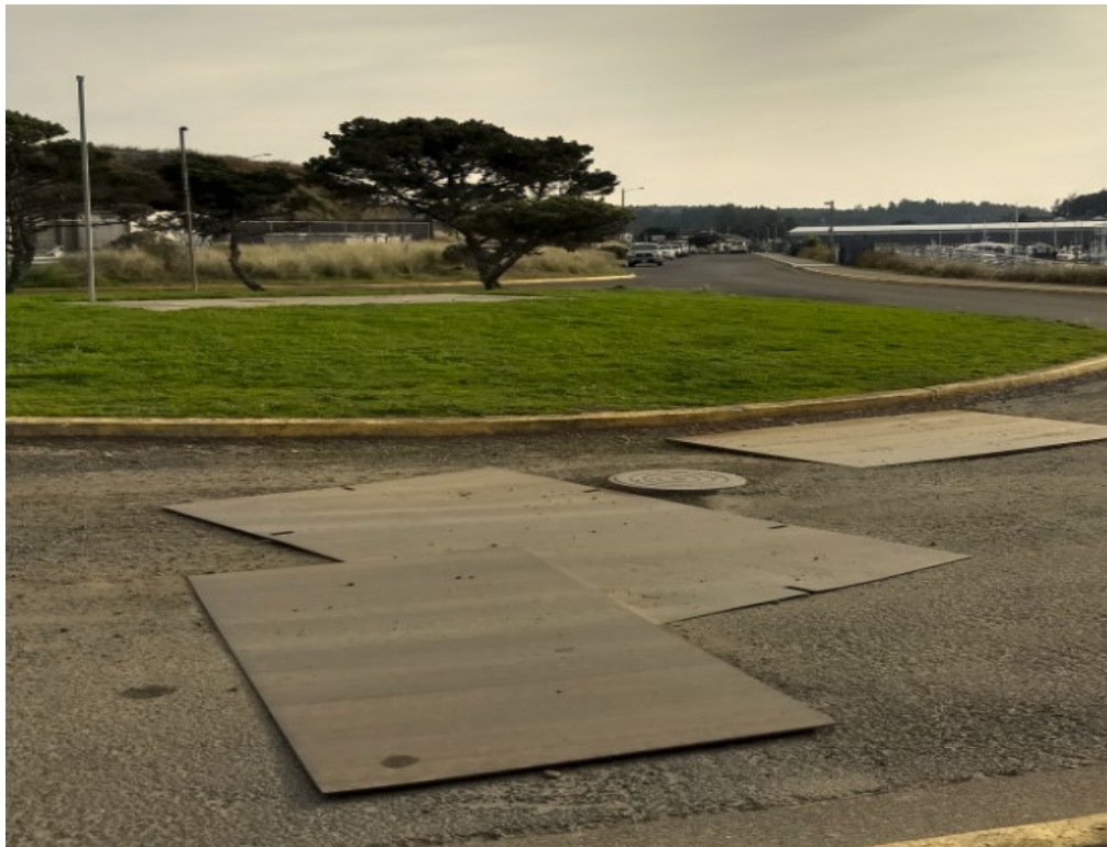
Photo 32 – Patched Road near Fuel Dock
