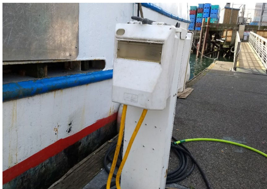
Photo 4 – Port Dock 3 – Electrical Pedestal
