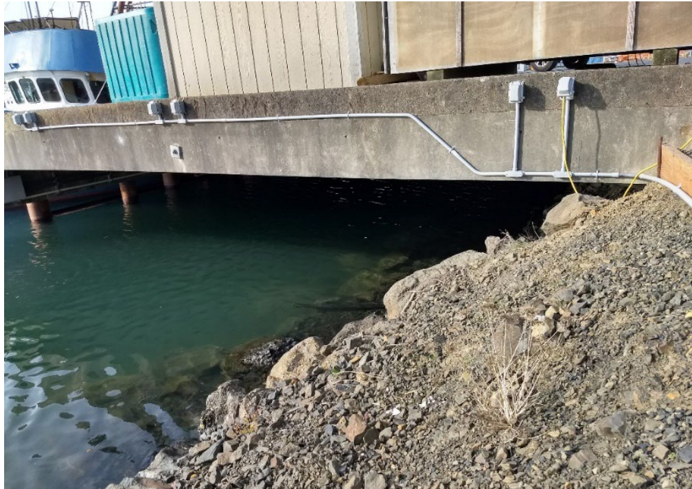
Photo 15 – Hoist Dock – Electrical in Tidal Zone
