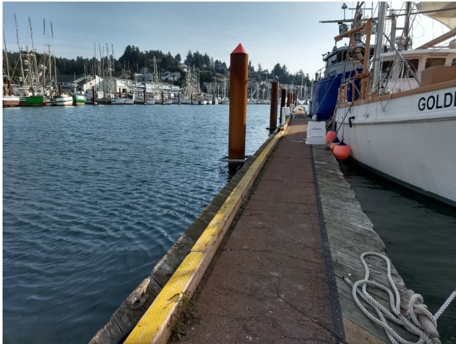
Photo 12 – Port Dock 7 – Floating Dock B
